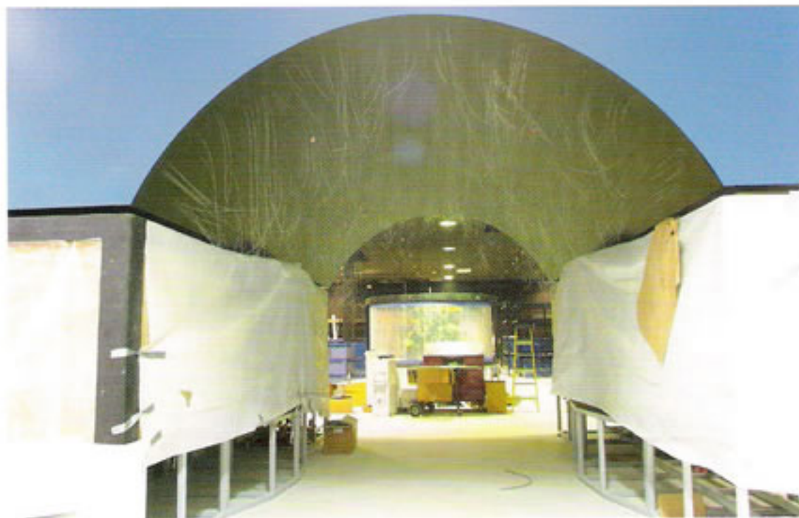
TUNNEL VISION: Big Al's Aquarium Supercenter will include an 8,000-gallon fiber-optic tunnel with freshwater and saltwater display tanks. Company photo
